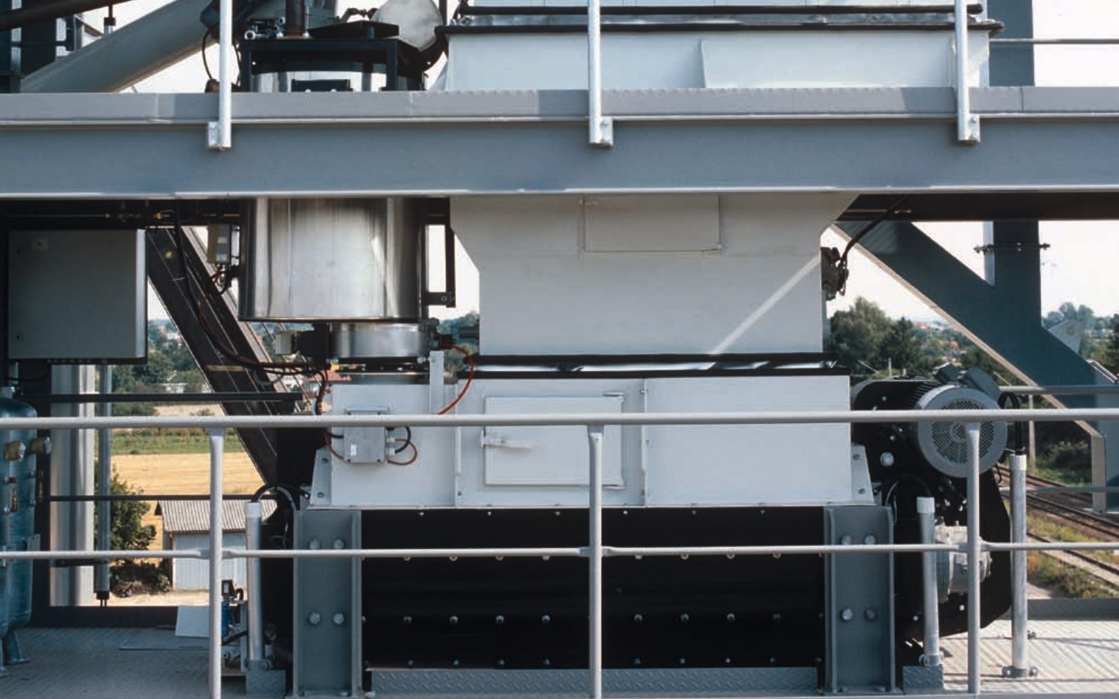
Weighing and mixing level with a 4-ton asphalt mixer
