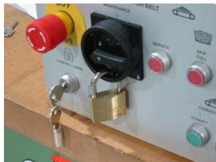
Figure III - 3: Maintenance switch with padlock
