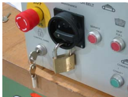
Figure VI - 1: Maintenance switch with padlock
