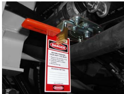
Figure VI - 2: Hydraulics maintenance switch
