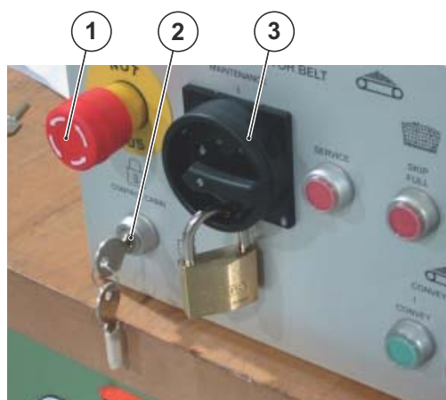
Figure III - 1: Emergency stop device on control panel
