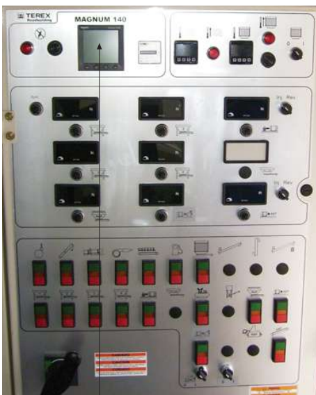
Panel de control manual
