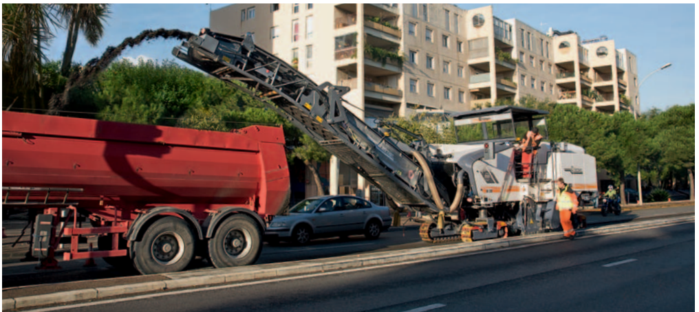
Cold milling machine being used for the rehabilitation of an inner-city asphalt surface course
