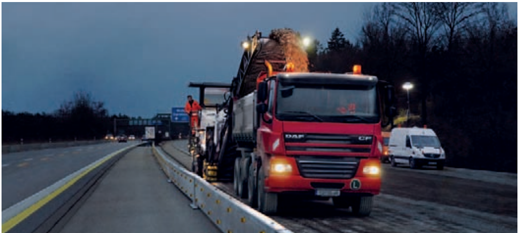
Cold milling machine being used for the rehabilitation of a main road at night
